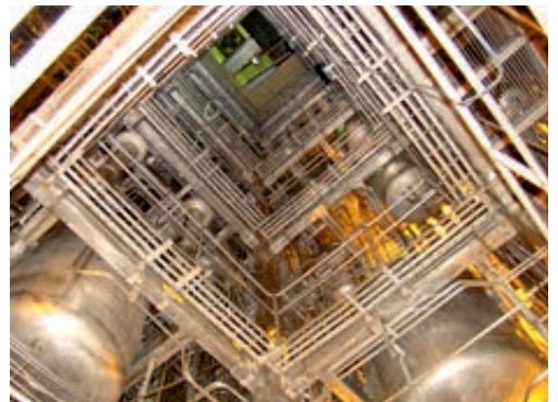
Inside view of hot cell of reprocessing plant KARP
