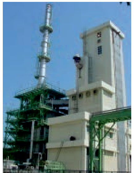
Steam Generator Test Facility
