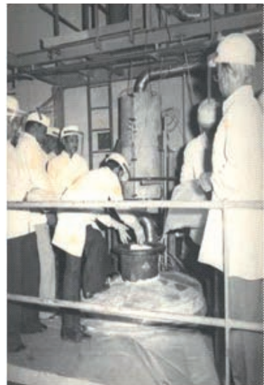
First Sodium Charging in melter tank for sodium purification for FBTR
