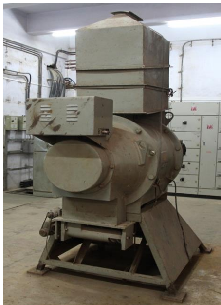
Fig. 1: A dry storage type grain irradiator with grain lifting conveyor system (collaboration with AECL, Canada, currently the facility is not in operational state).
