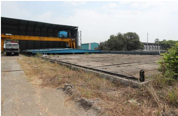
Reinforced Concrete Trenches (RCT)
