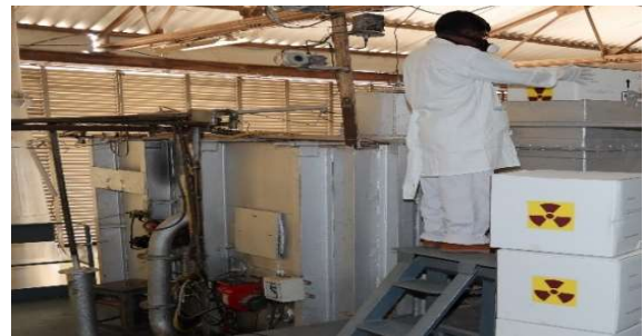
INCINERATION SYSTEM Volume Reduction Factor: > 30
