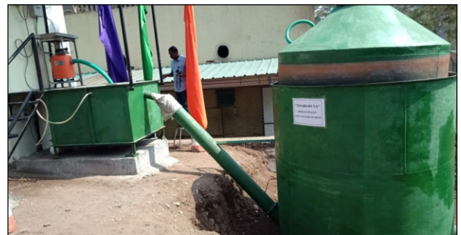
Fig.4: Nisargruna plant at CISF Headquarter, BARC.
