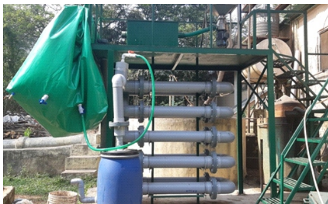
Fig. 4: Shesha pilot plant installed at Training School Hostel during 2021.
