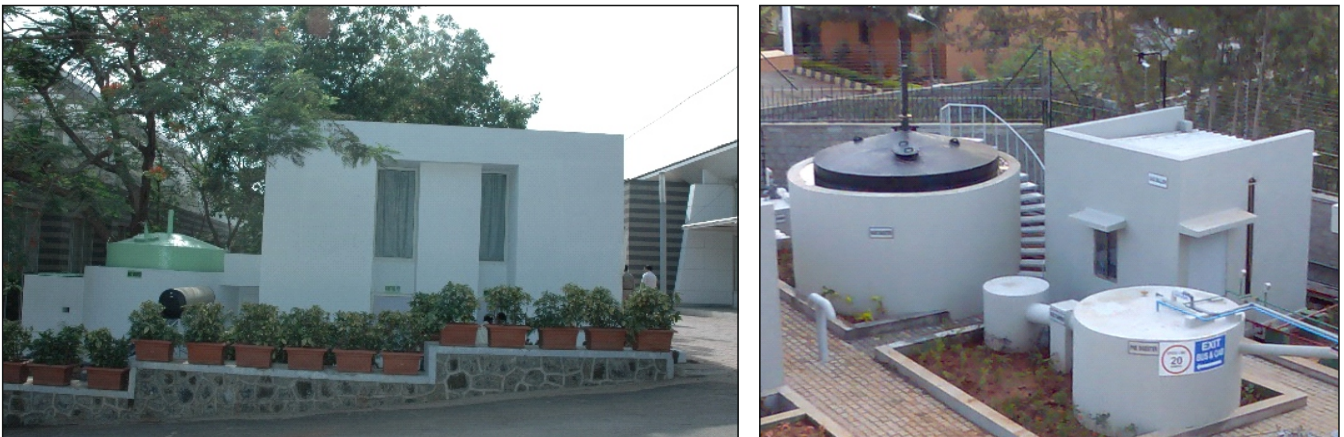
Fig.7: Nisargruna plant at TCS, Thane and Wipro, Kochi.
