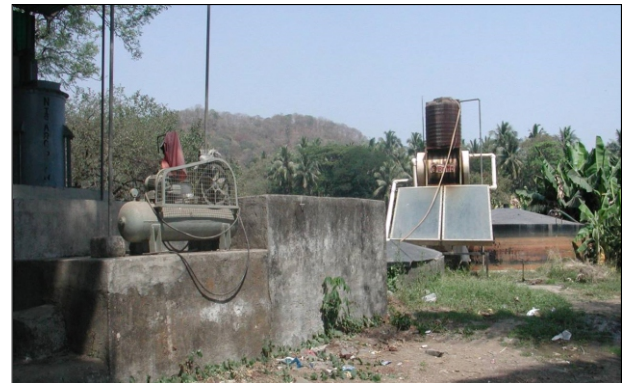
Photo.1: First Nisargruna plant installed at Nursery, BARC 2001.
