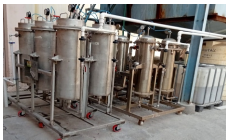
Textile Effluent Decoloration treatment plant (75KLD) installed at Jodhpur (Top).
