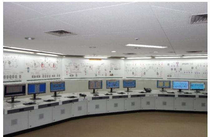
Upgraded PLC-SCADA System of WIP Trombay.
