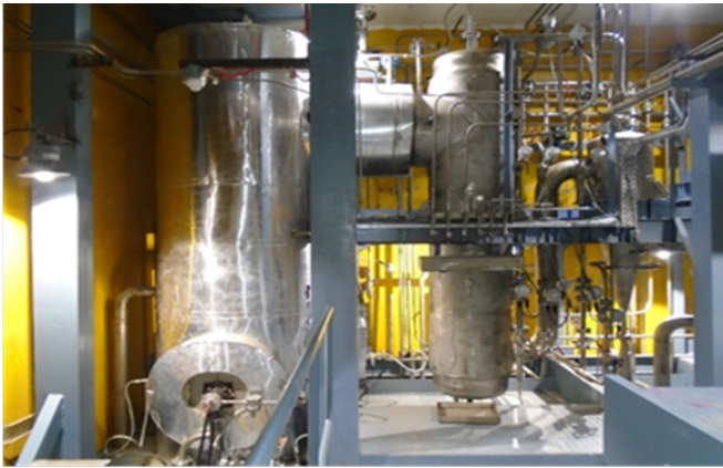
Incinerator (left) & Quencher (right) of Organic Liquid Waste Incineration System (OLWIS).
