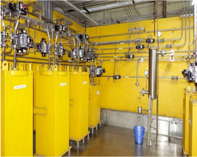
The Effluent polishing system at WIP Trombay.
