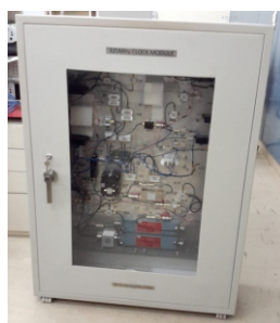
325 MHz Reference phase generation system.
