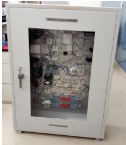
Fig.1: 325 MHz reference phase generation system.
