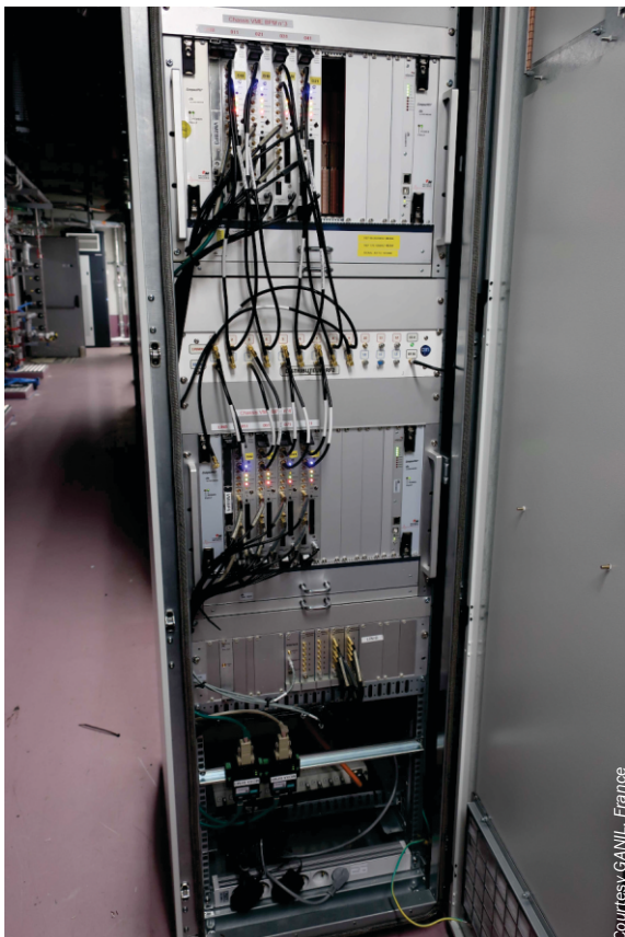
Fig.15: 8 of the 20 BPM modules at SPIRAL2 LINAC tunnel.
