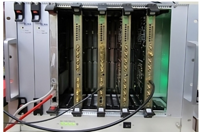
Fig.7: One RFPI system with four VME modules.
