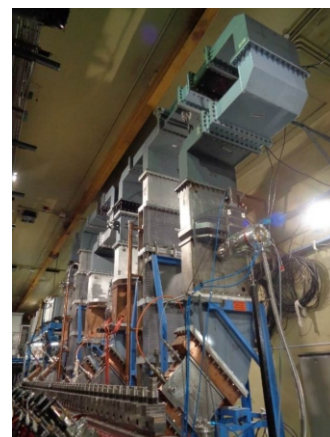
Fig.6: Installed and commissioned waveguide systems of 10 MeV DTL.
