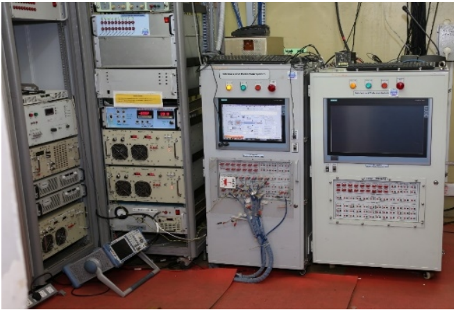
Fig.3: Interlock and protections systems and LV supplies.
