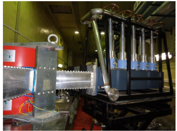
Fig.4: Circulator (1 MW) and 0.8 MW RF Load.
