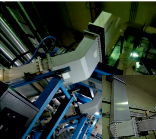
Fig.5: Waveguide transmission line from Klystron HPRF to 3 MeV RFQ.
