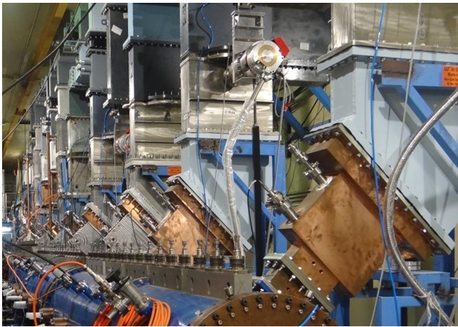
Fig.7: Installed and commissioned waveguide systems of 20 MeV.
