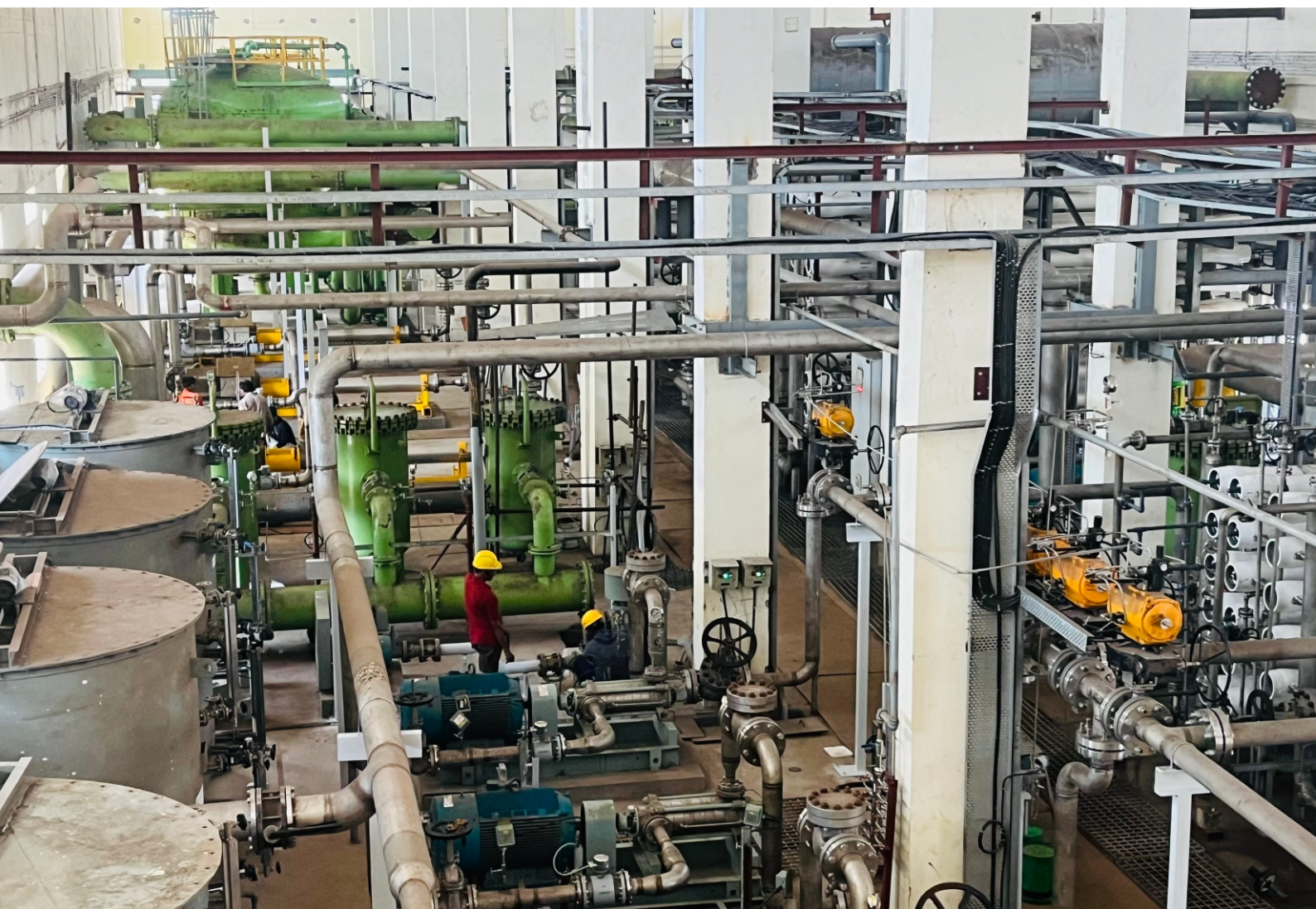
Inside view of Seawater Desalination Plant equipped with BARC Technology commissioned at OSCOM in Odisha.
