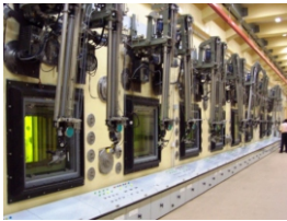
RDMs installed in hotcell
