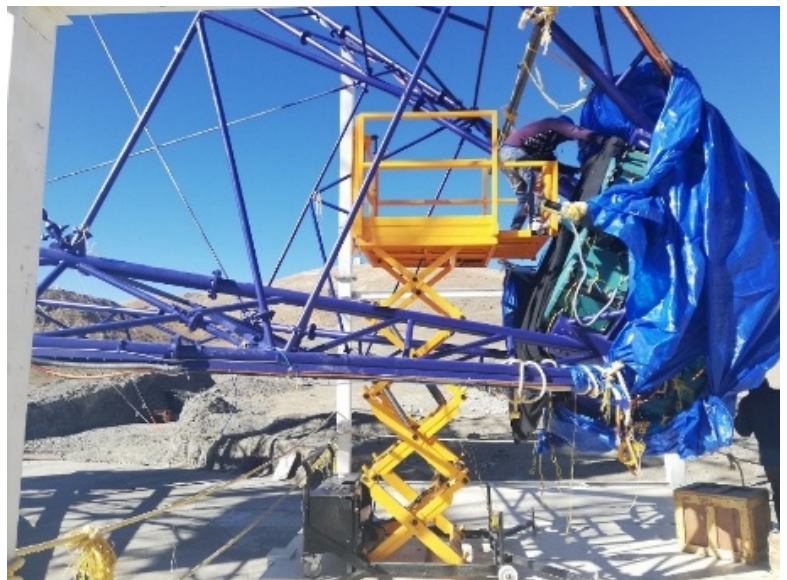
▲ AERIAL Work Platform for Camera module access.
