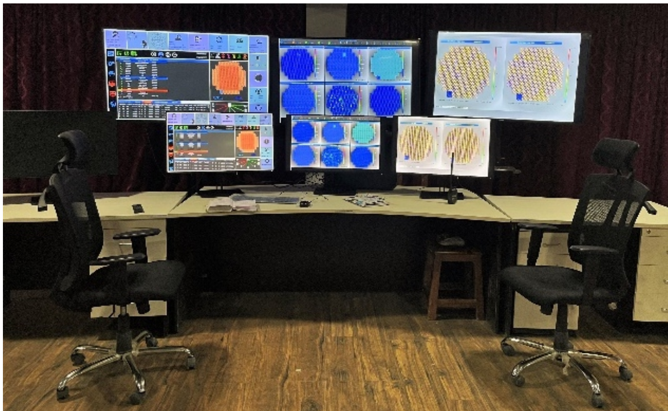
▲ MACE Control Room Setup at Hanle.
