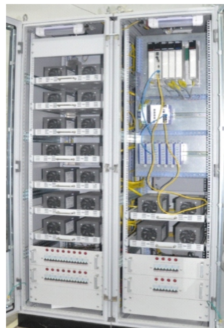
▼ POWER Supply rack.
