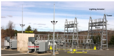
Typical Electrical Substation of a Nuclear Facility
