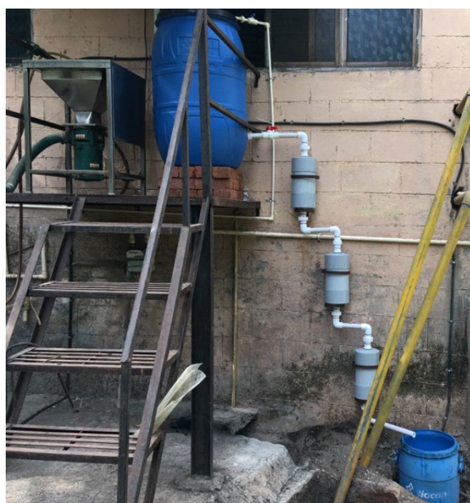
Fig.2: Pilot scale facility installed at BARC Training School Building, Anushaktinagar, Mumbai.
