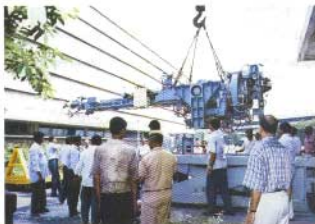
Fuelling Machine being unloaded from service cart on way to Project stores, NPCIL.
