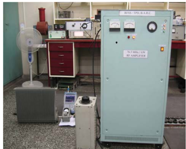
Fig.3: Photograph of 1 kW, 76.58 MHz RF system
