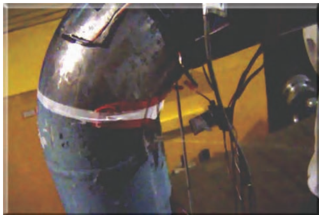
Fig. 37: Failure of piping system
