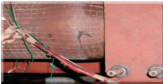
Fig. 31: Bulging of pipe
