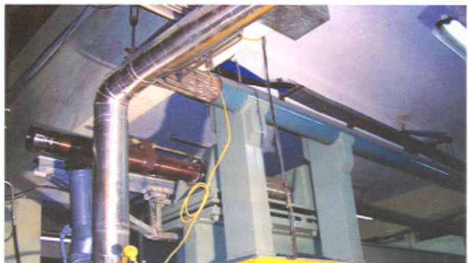
Fig. 1: Coolant channel of 540 MWe PHWR
