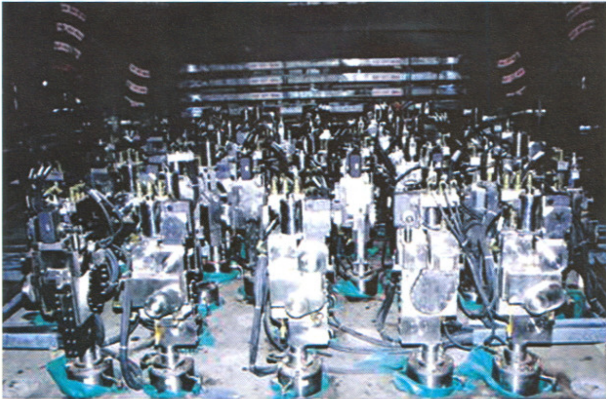
Photograph showing reactivity control mechanisms on desk plate of TAPS 4 reactor
