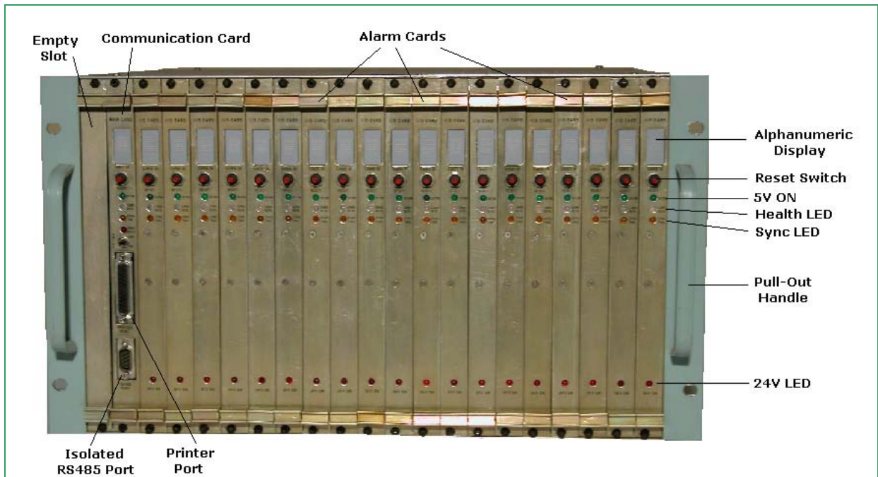
Alarm Annunciation System - Front View
