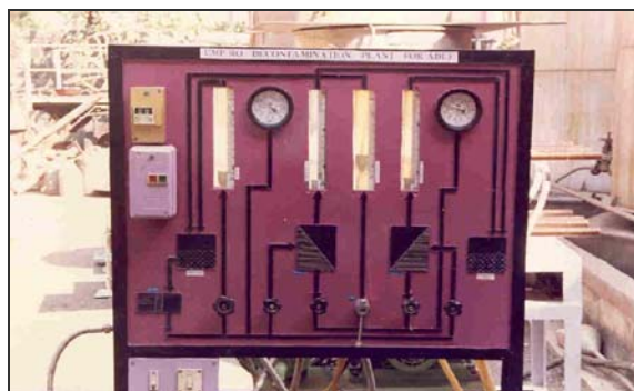
RO plant for effluent treatment in uranium metal plant (UMP)
