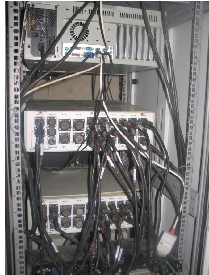
Controller -BACK view
