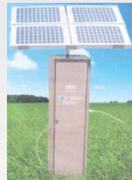
RO/UF Unit with PV Panels
