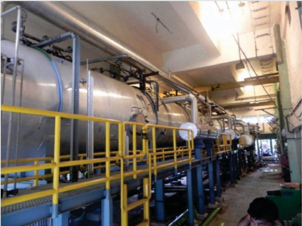
240 m 3 /day MED-TVC Plant at DD, BARC, Mumbai
