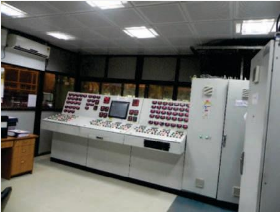
Operator Desk of MED-TVC Plant
