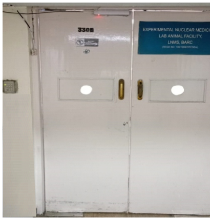
Fig.4: Electronic Door Lock: Access control door lock facility for animal house main entrance door.
