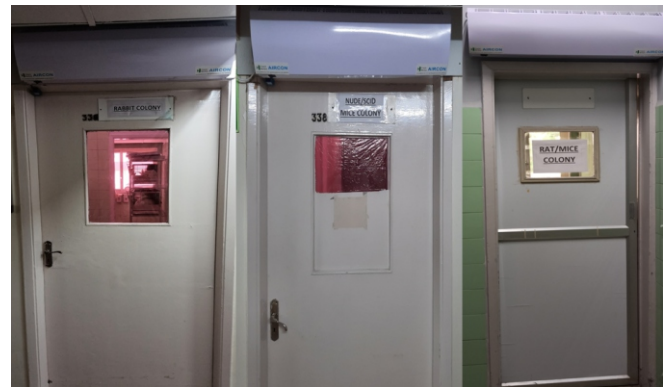
Fig.11: Air Lock System: Animal colony with air curtain and limit switch at entry door.
