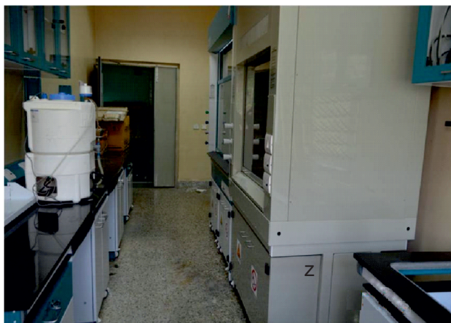
Fig.3: Chemical laboratory in CTL, TPD showing installed fume hoods, water purifier, racks and working table.
