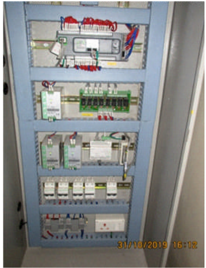
Fig.5: Pp1 Communication Chamber
