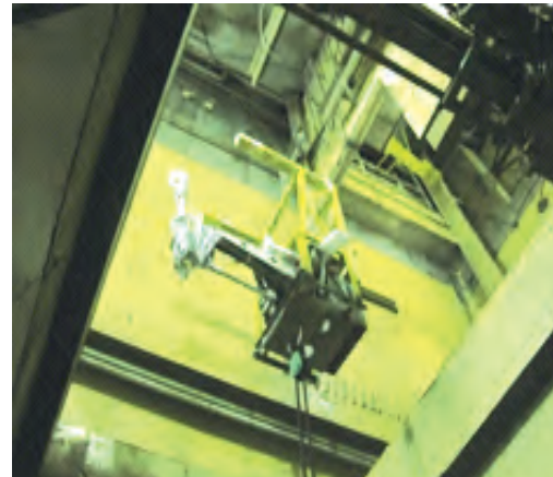
Lowering arm in Vitrification cell
