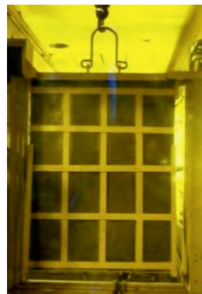
Figure 7. Portable lead shielding mounted on the cut out of wall between Melter cell and Installation site
