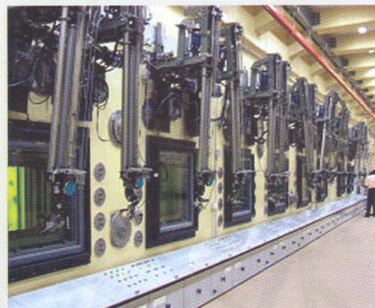
RDMs installed at PIED hotcell
