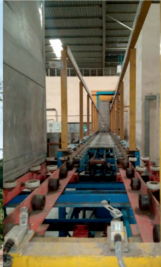
Inside view of Ahmedabad Sludge Hygienisation Plant.
