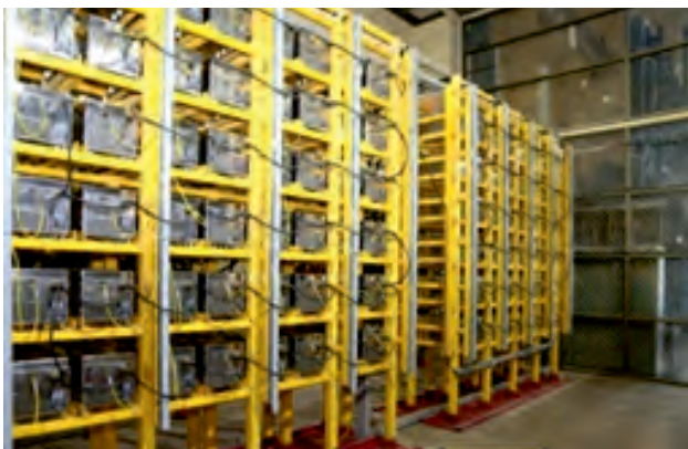
RHVPS sub-system commissioned at LEHIPA.
