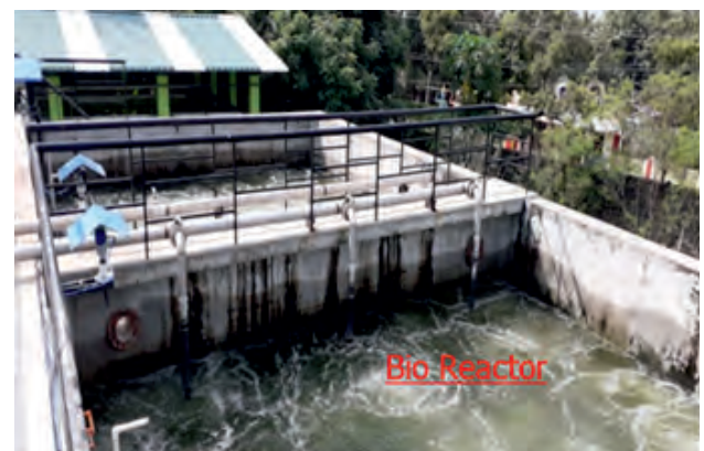
The 1.5 MLD hgSBR based Sewage Treatment Plant (STP) in DAE Township, Kalpakkam.
