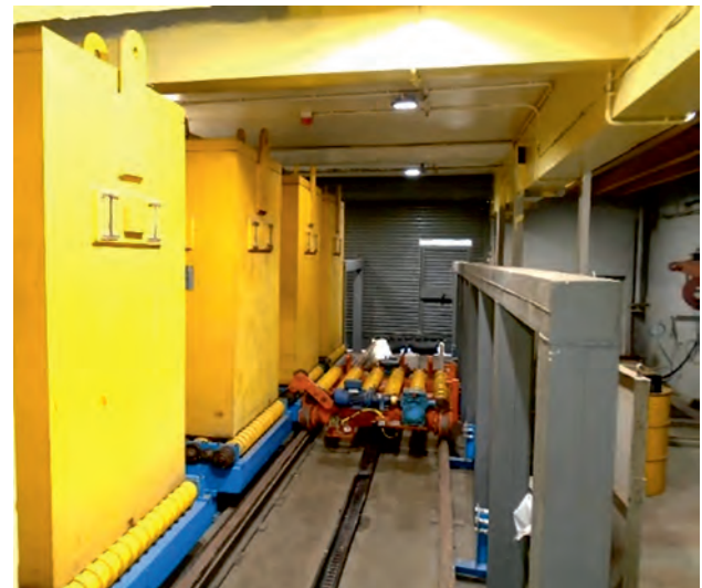
Ion Exchange (IX) Plant at ETP in BARC.
