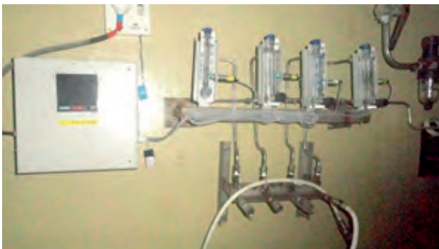
Low Flow Based Alarm System for Fresh Airline Manifolds.
