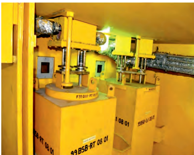
Ion Exchange columns at PHIX System.
