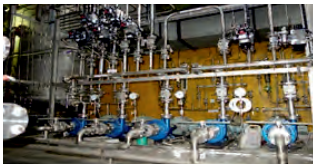
Effluent Conditioning and Transfer System at WIP in BARC.
