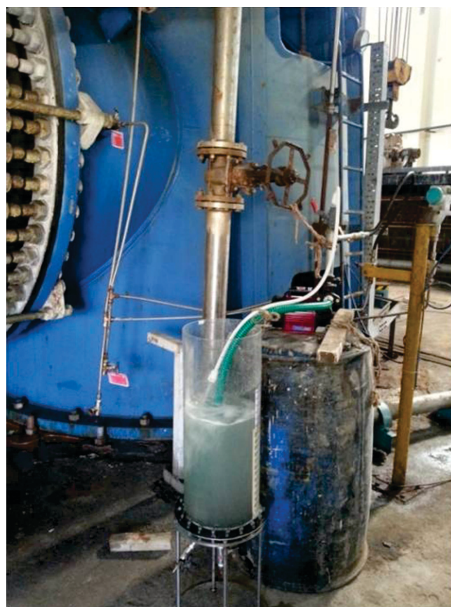
Fig.10: Injection system used of injecting the radiotracer into the pipeline
