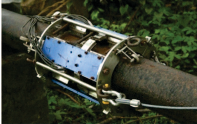
Fig. 4: EPIG over the discharge pipeline at IF3 BARC
