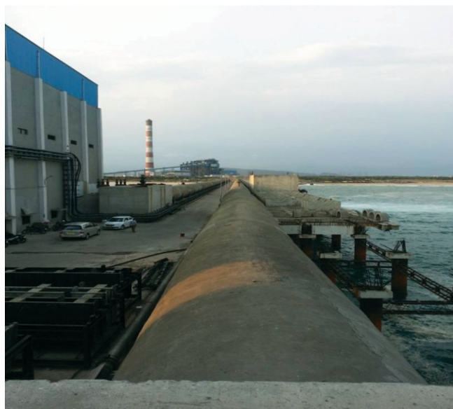
Fig. 8: Large diameter pipelines used for transporting the cooling water
