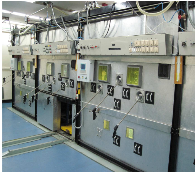
Fig.2: 100 mm lead-shielded isotope processing plant for radiochemical processing of 177 Lu at IP & AD, BARC
