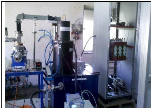
Fig. 10: Modulator with single-beam klystron on test
