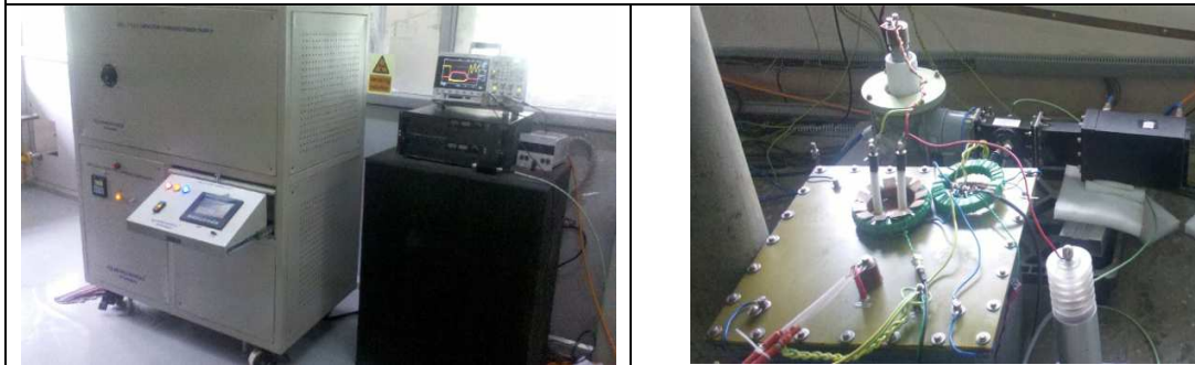
Fig. 2: View of Magnetron Modulator and Pulse Transformer Tank
