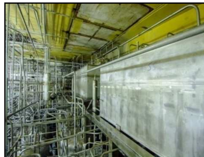
Fig.5: In cell view of cesium separation facility at WIP, Trombay
