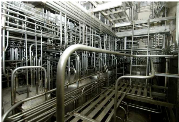
Fig. 2: Actinide Separation Demonstration Facility, BARC, Tarapur
