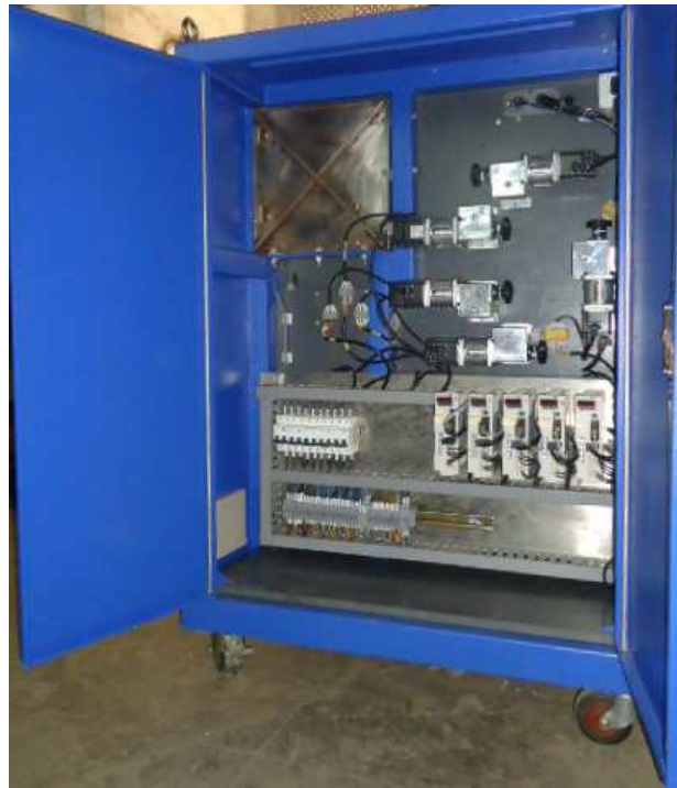
Fig. 3: Photograph of the electronic drive and control systems of the MROD. There are two sets of electronic drive control systems mounted left and right sides of the device. Only one side is visible in this photograph
