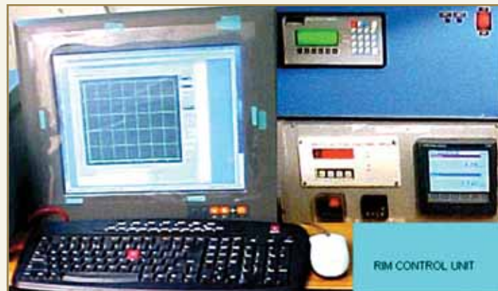
Fig. 7: Control station for ID measurement system
