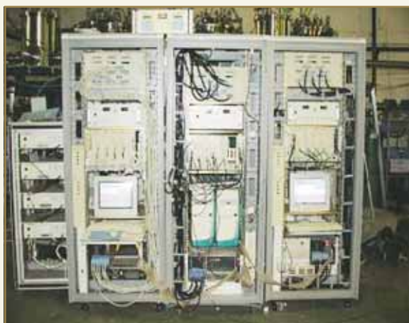
Fig. 4: Control electronics modules installed at TIFR for the control of 3 cryostats
