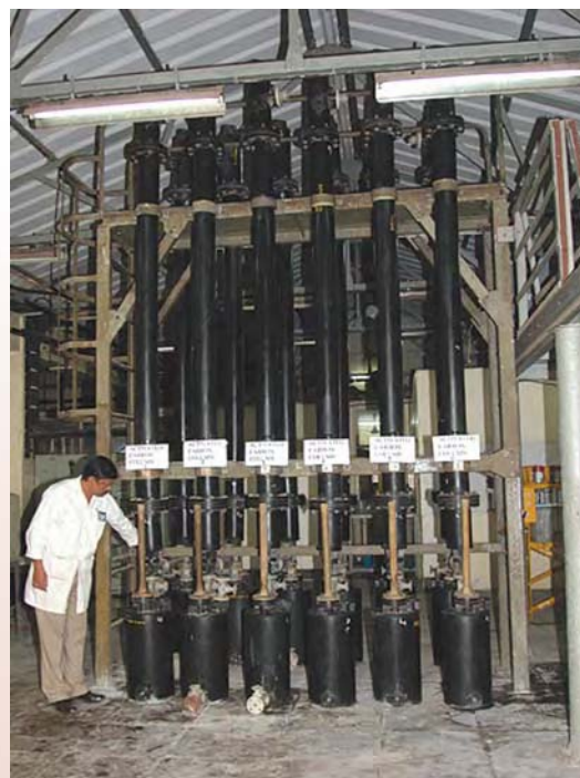
Fig. 2: Photograph of carbon columns for pre-treatment
